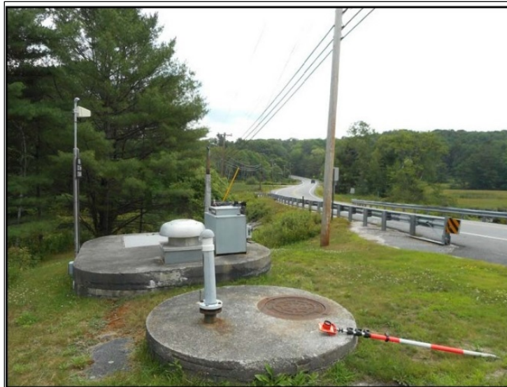
Figure 1: Mast Landing Pump Station
