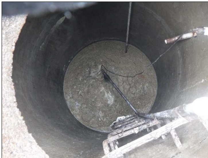
Figure 2: FOG Buildup - 2 weeks after cleaning the well (Pre-Trial) – 1-25-17
