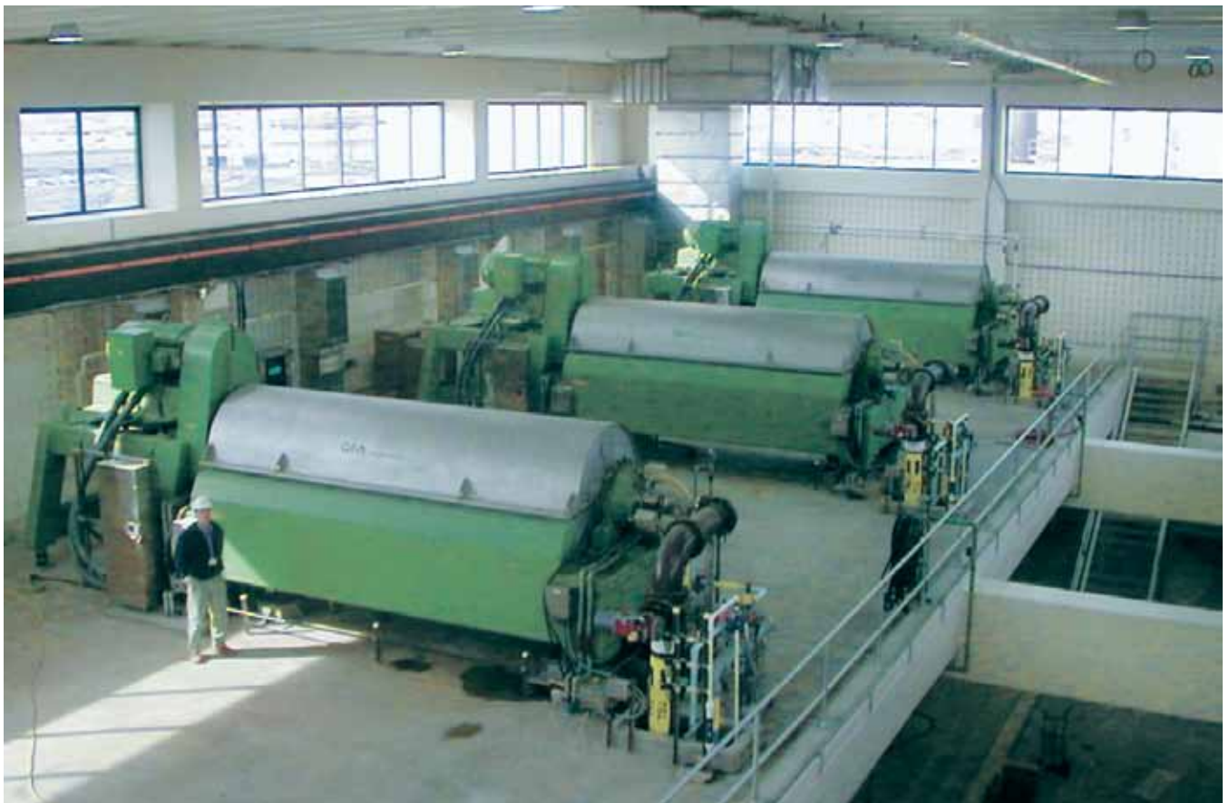
The PVSC water resource recovery facility uses four thickening centrifuges that play a critical role in its solids treatment train. PVSC
