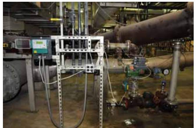
A full-scale test program of the new meter, left, was conducted on one centrifuge. PVSC
